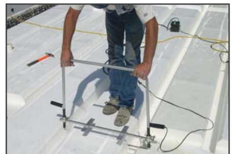
Cutting into Quad-Deck panels is quick and easy with a hot wire
